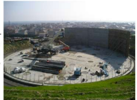
3MG Pre-Stressed Concrete Tank
