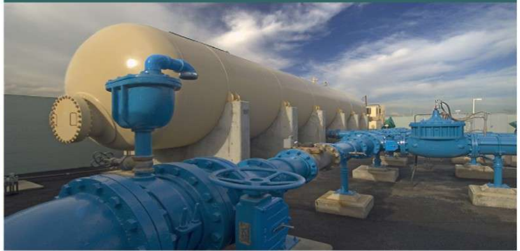
Municipal Booster Pump Station
