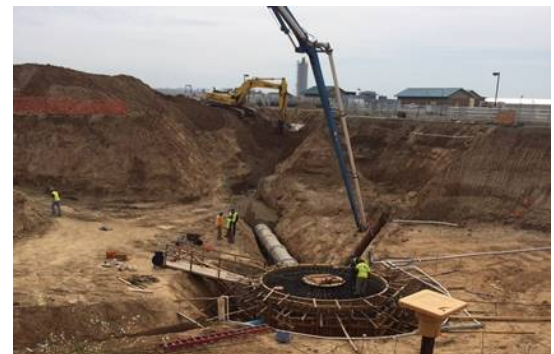
Mid-Western Placer Regional Sewer Project, Placer County: "Construction of new 108' diameter clarifier at Lincoln Wastewater Treatment and Reclamation Facility."
