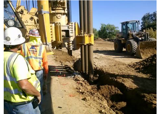
Feather River West Levee Rehabilitation Project, Sutter County: "Deep Mix Slurry Wall Construction"
