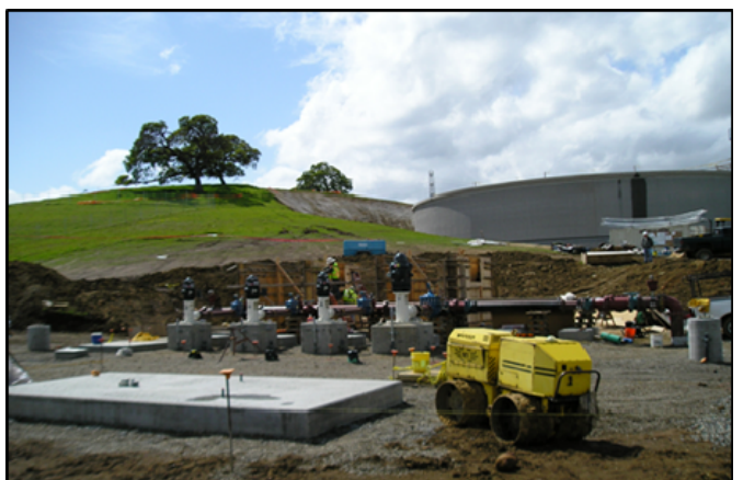
4 MG Vineyard Tank and Pump Station Shea Homes, Brentwood, CA
